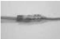
Orange wire connection
